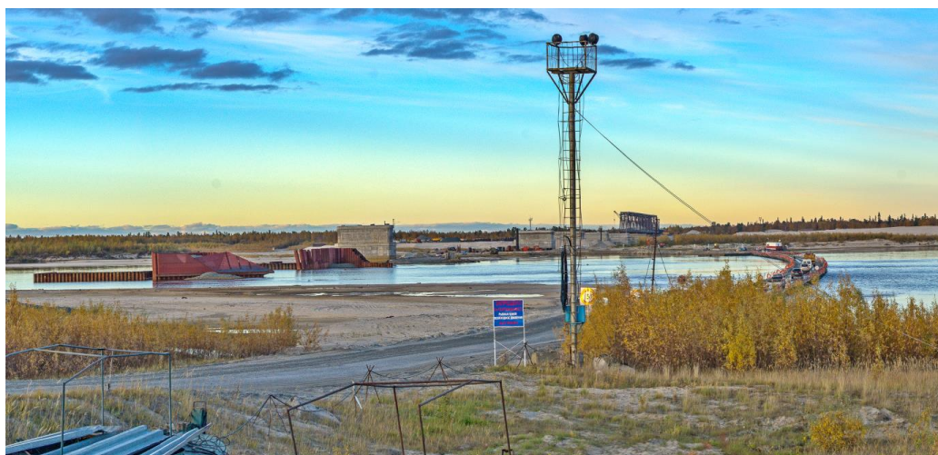
Fig. 9. Pontoon crossing and the start of construction of the road bridge across the Nadym River (photo by O.S. Sizov, 2012).
